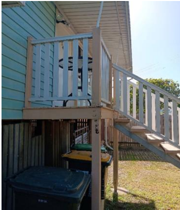
Minor. The front southern balcony is out of level subject to the age of the property. Recommend a builder to replace or rectify as required.
