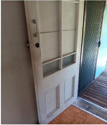
General deterioration to the rear door.
