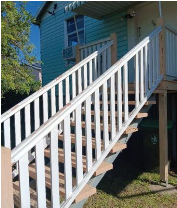
Minor. The front verandah handrails require fixing by a builder.
