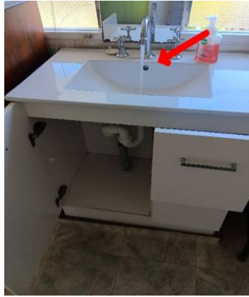
Bathroom Vanity. No water leaks were found inside the cabinet on the day of inspection. Please note, the red arrow shows the water running for water leak inspection. (This was dry on the day of inspection.)
