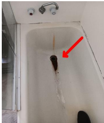
Major. Rust to the bath. Recommend a builder to replace.
