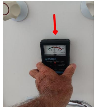
Moisture Readings Found- Major Defect. Major moisture readings were found as per the photo supplied, after using a tramex plus moisture unit. There is a high possibility of structural internal wall framing damage. Recommend a plumber or a builder to do an invasive inspection and rectify the problem. Receipt of repairs is required for the buyer, stating they have fixed this problem.
