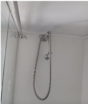
Minor. The shower rose fitting requires replacing by a plumber.
