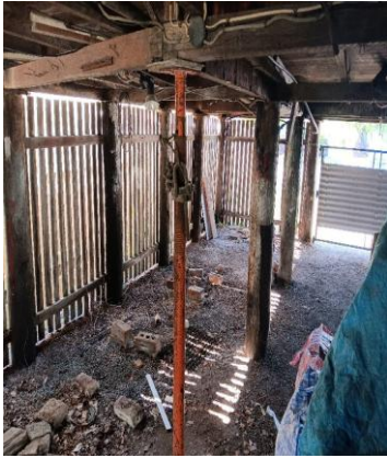
Major Structural. All the timber stumps require replacing by a builder.
