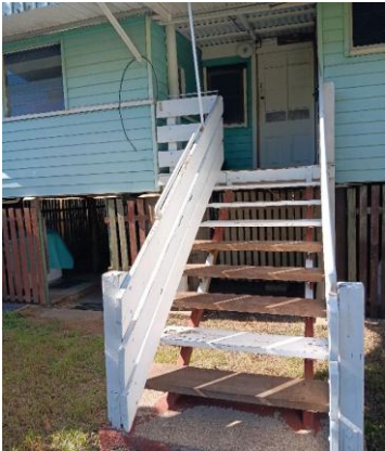
Rear Northern Steps. General wood decay to the timbers. Recommend a builder to replace as required.
