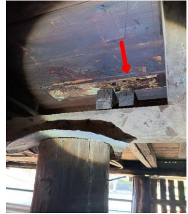
Minor. Borers to the floor in several sections of the floor. Please read the report by the pest inspector.
